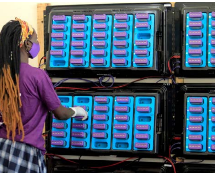
VAC Solar is establishing solar hubs and a distribution network for rental battery packs in Uganda.
